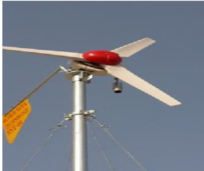
FIGURE 3. 0.7 kW SNT-1 rooftop wind turbine installed at GERMI rooftop
