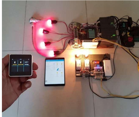
FIGURE 2. IOT based Industrial Automation
