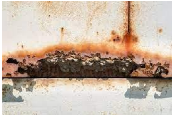
FIGURE 1. Stress Corrosion Cracking
